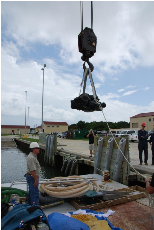
US Coast Guard crane operators removing the sounding weight concretion from Jones Bay .
